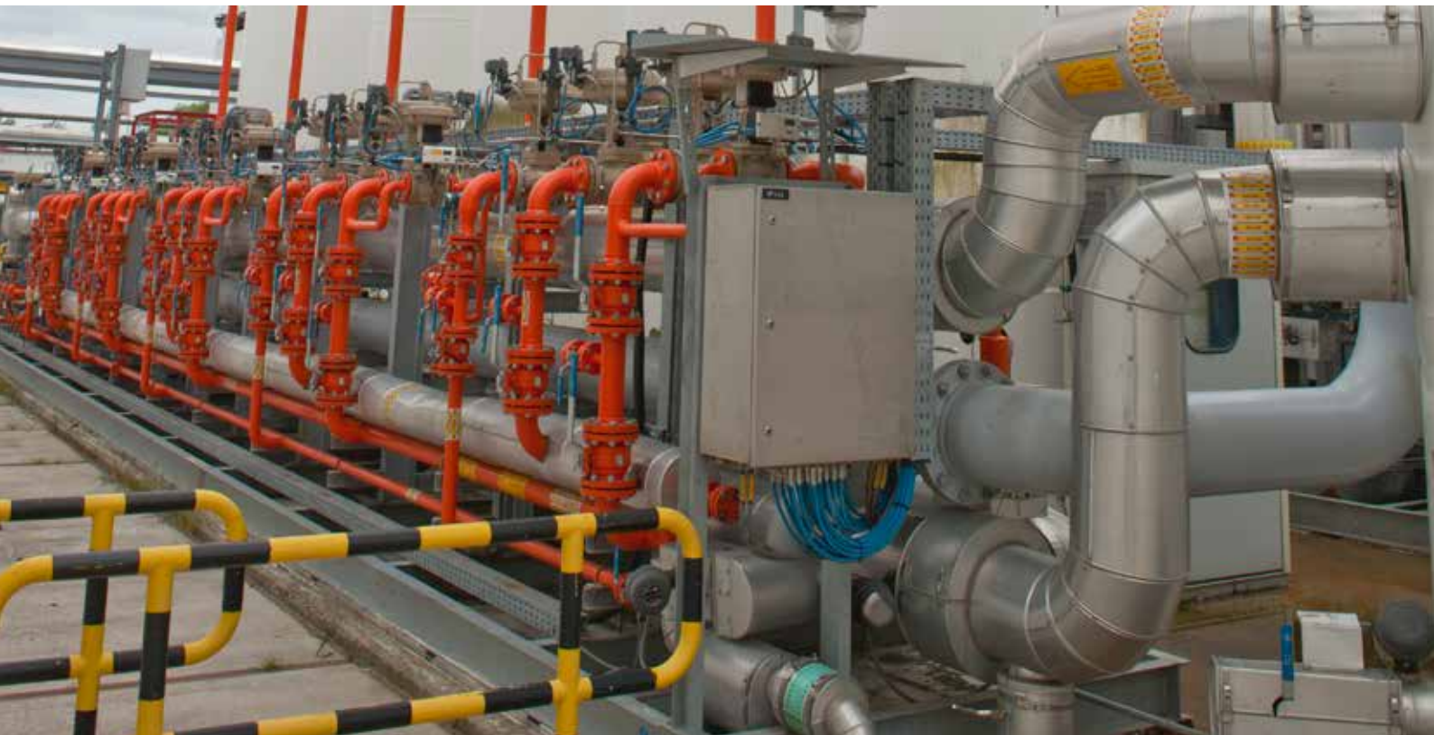
PSA unit for hydrogen purification in the Netherlands
