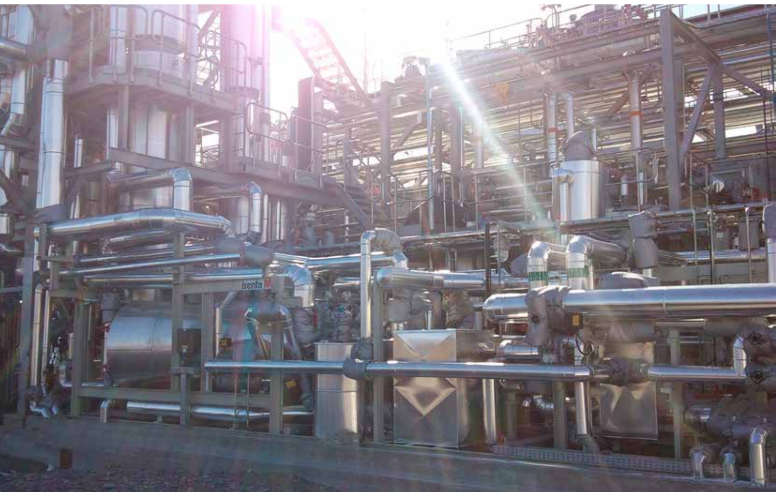
CO 2 removal within bio DME demonstration plant
