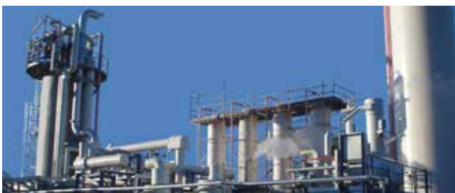
Start-up of the plant
