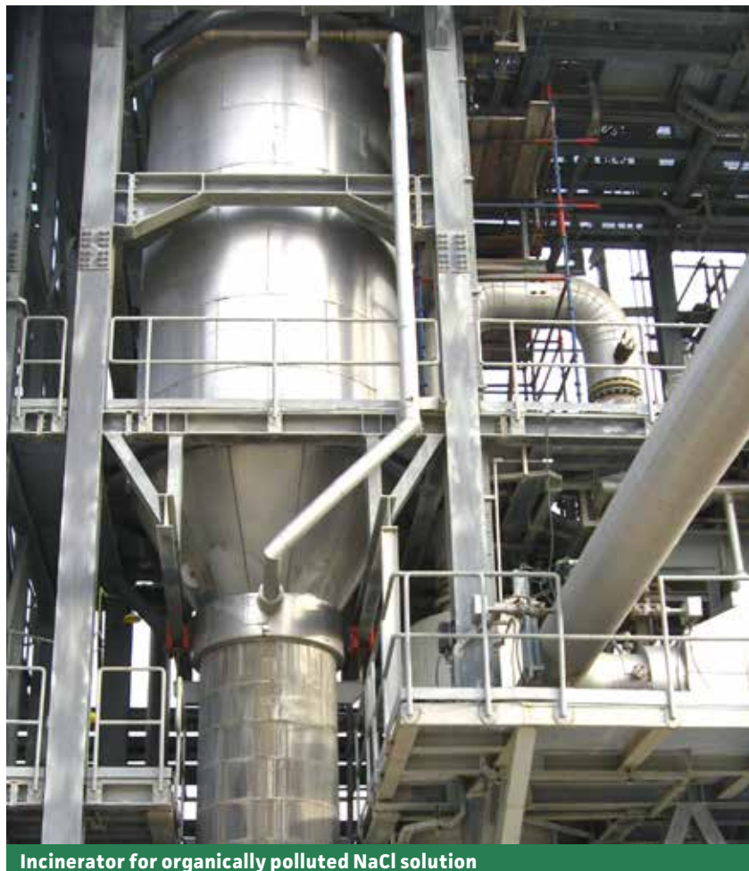
Incinerator for disposing organic polluted NaCl solution
