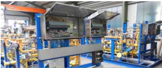
Factory acceptance test in CALORIC's production facility
