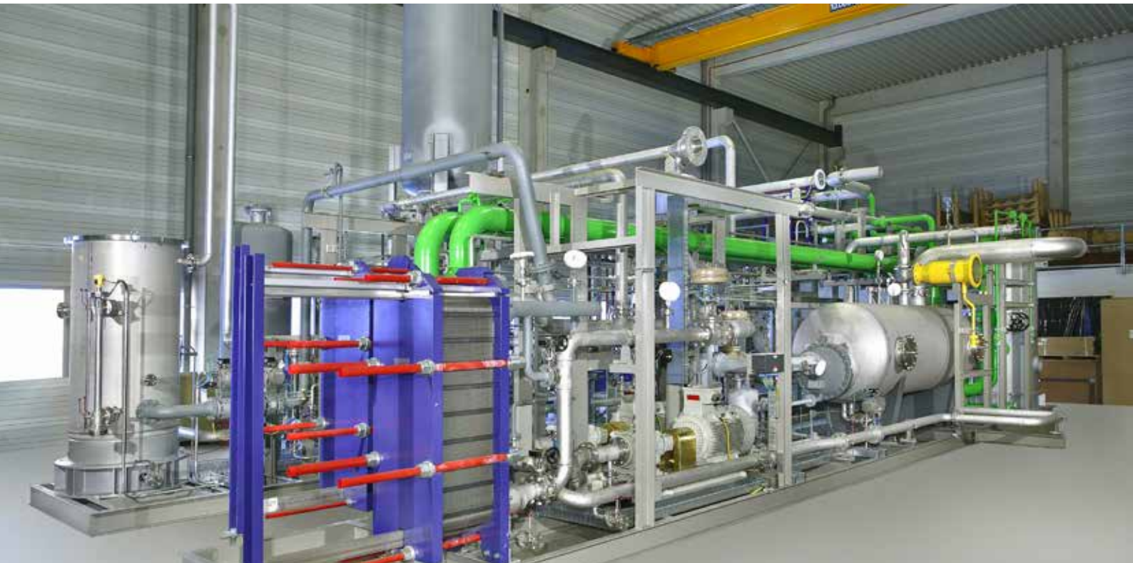
Amine recovery skid during manufacturing
