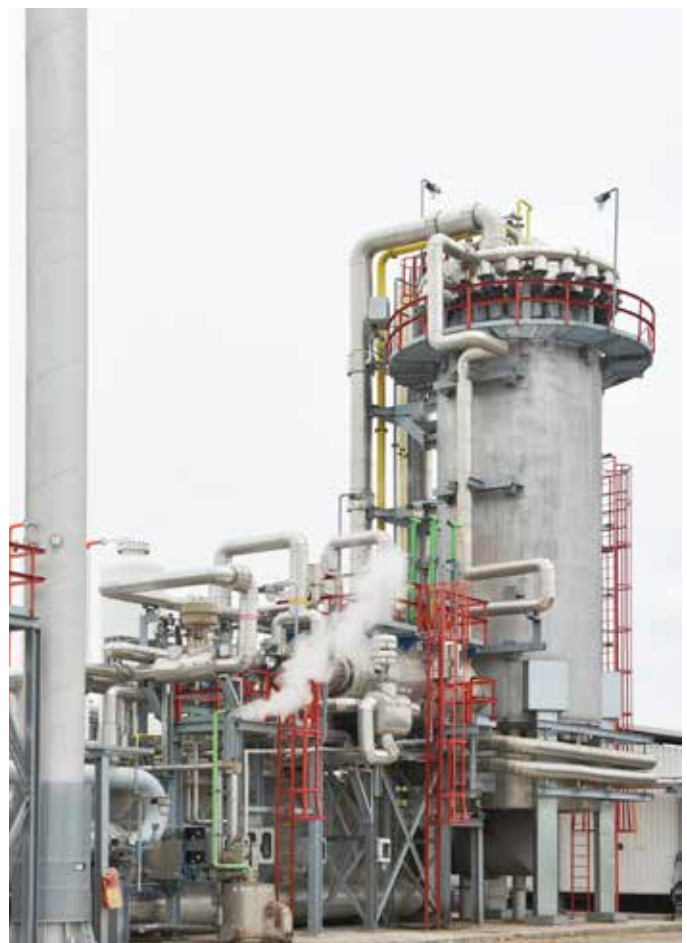
Steam reformer for 4000 Nm 3 /h hydrogen (purity 99,9%)
