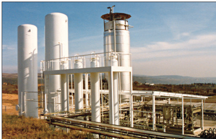
A methanol reformer with a pressure-swing-adsorption unit.
