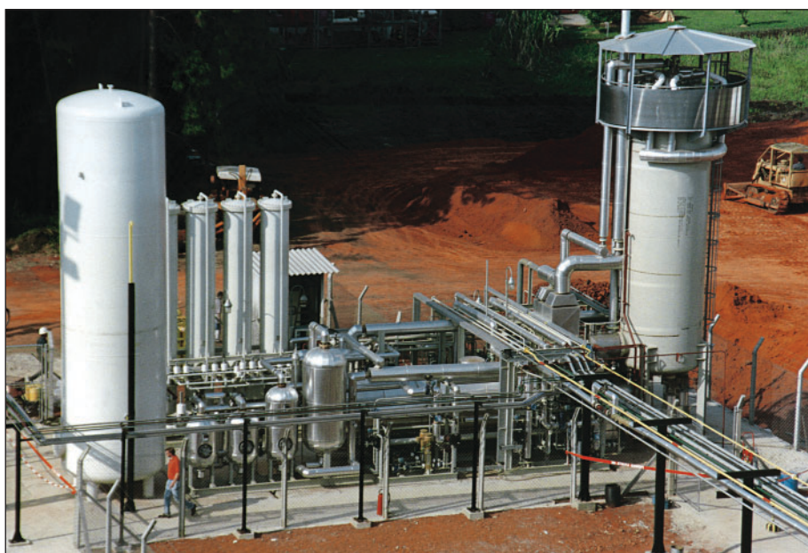
A steam reformer with a pressure-swing-adsorption unit.
