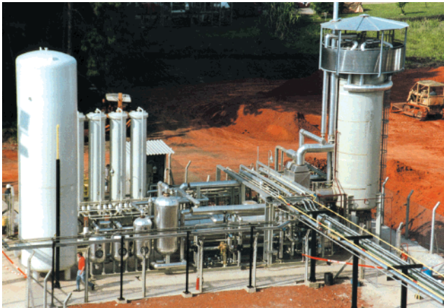
Figure 4. HC steam reforming plant with a capacity of 500 m 3 /h hydrogen supply
