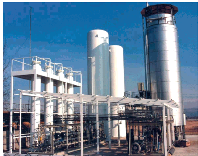
Figure 2. Methanol reforming plant with a capacity of 500 m 3 /h hydrogen supply
