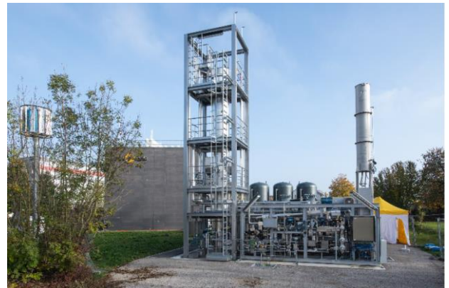
Fig. 2: Biological methanation plant ©RES
