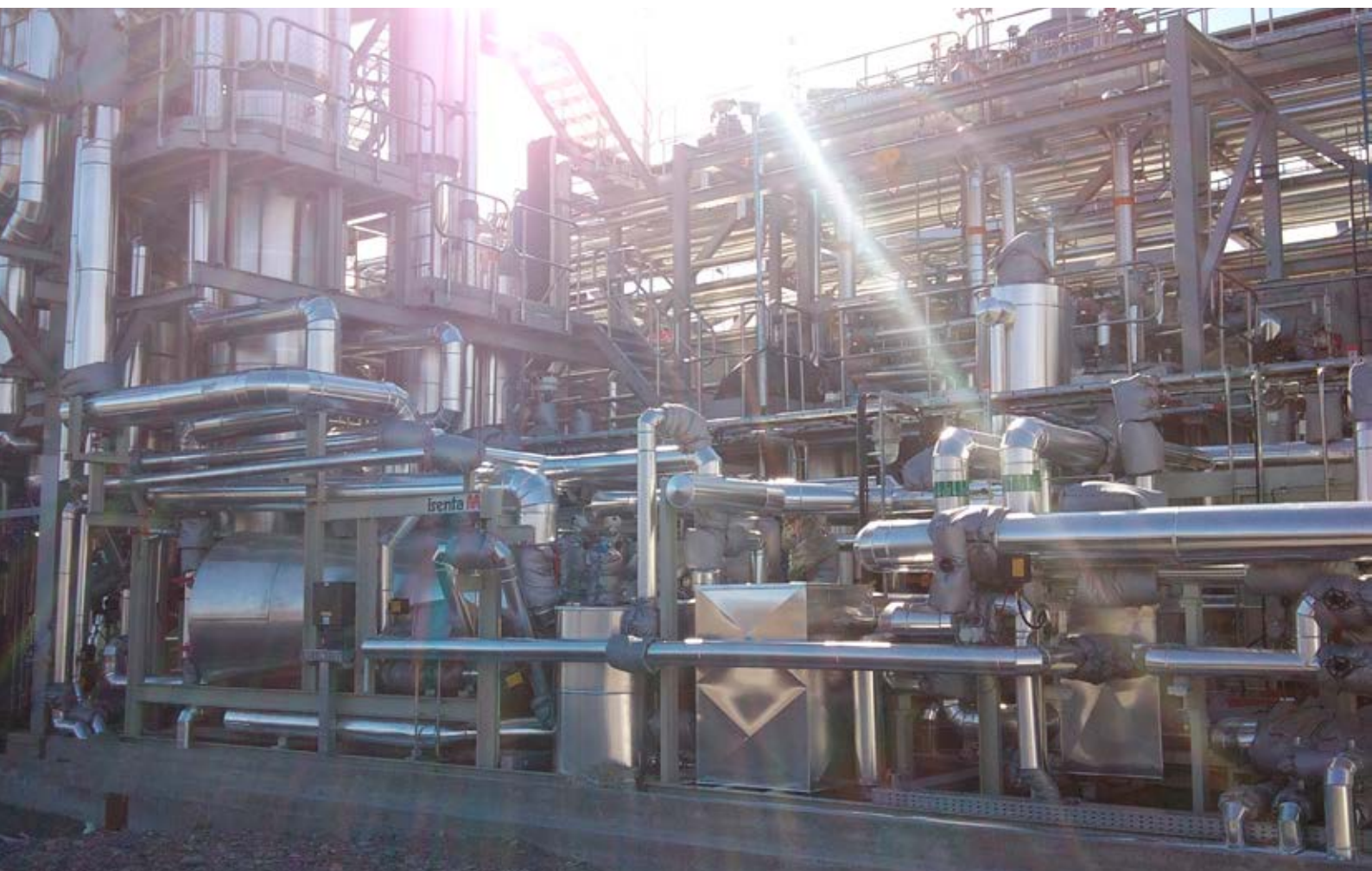
CO 2 removal within bio DME demonstration plant
