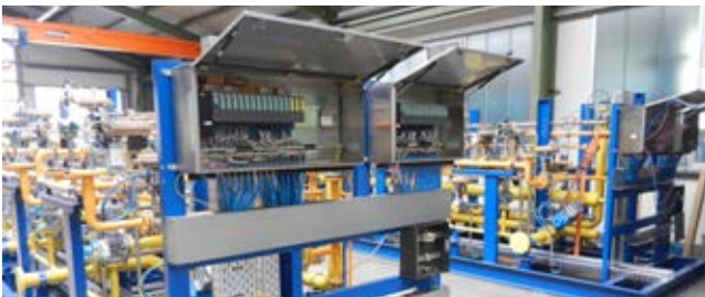
Factory acceptance test in CALORIC's production facility
