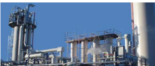
Start-up of the plant
