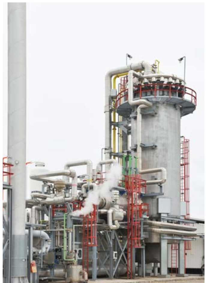
Steam reformer for 4000 Nm 3 /h hydrogen (purity 99,9%)
